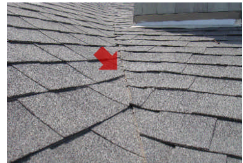
Debris & moisture becomes trapped.
