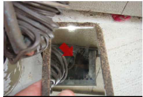
Seal void at the line set wall flashing.
