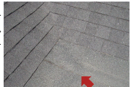
Suspect leak area, no bond to deck.
