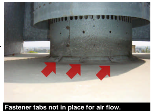
Fastener tabs not in place for air flow.
