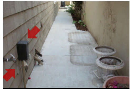
Covered J. box & low voltage light timer.
