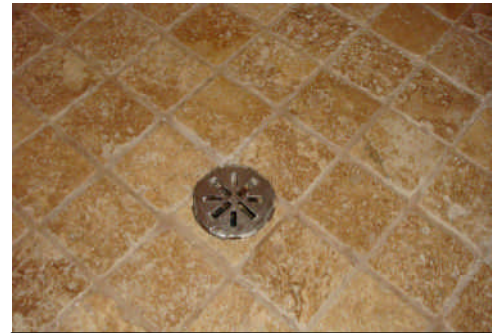
Second floor 3/4 shower loose drain cover.
