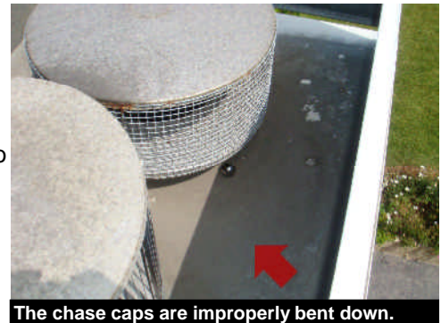
The chase caps are improperly bent down.
