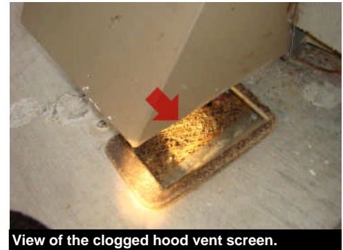
View of the clogged hood vent screen.
