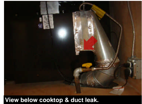
View below cooktop & duct leak.
