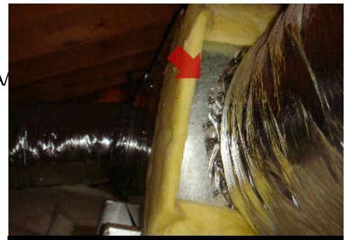
Un-insulated area of the cabinet.
