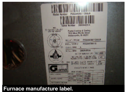
Furnace manufacture label.
