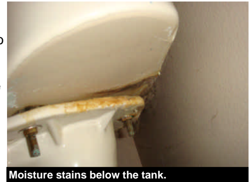
Moisture stains below the tank.
