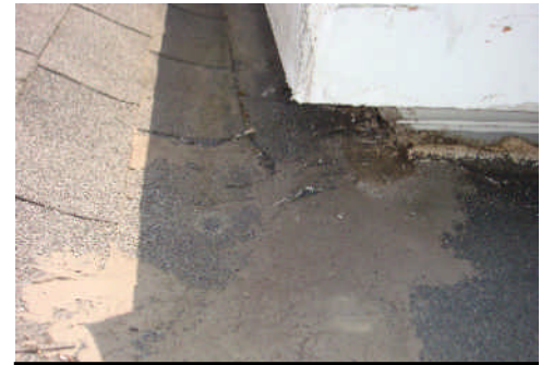
Patching will not correct conditions.
